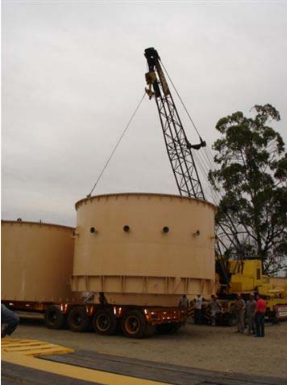
CPT column bottom section being loaded, nozzles for cavitation tube spargers are visible
