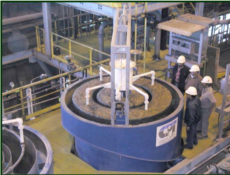
Figure 2: Wash water addition improves concentrate quality
