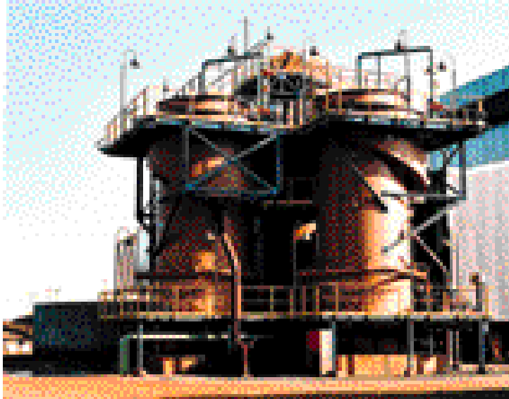
Figure 3: Column flotation plants are inexpensive and compact.
